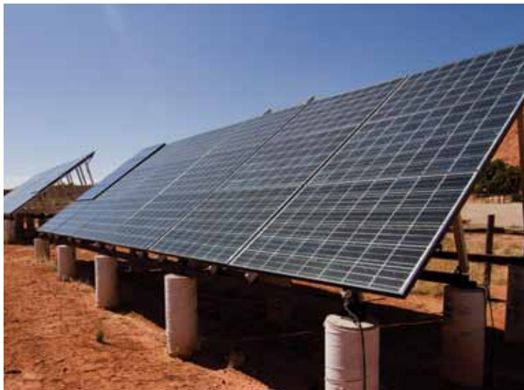
Solar panels in the Devils Garden Campground (photo by Andrew Kuhn)
